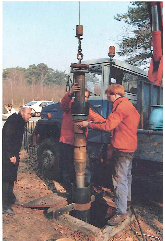
Fig. 13: Installation of the submersible pump into the pump jacket already moved down into the borehole.
