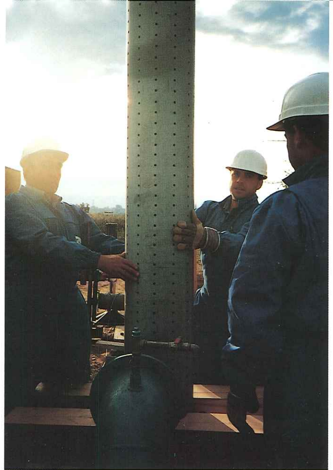
Fig. 11: Mounting of an SFCD-controlling pipe element.
